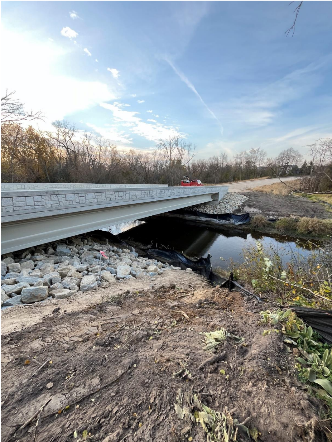
Parapet rock wall after sanding and grinding (touch up work and staining to occur in the spring).
