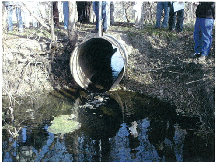
Image 16 – Existing culvert, raised in channel due to erosion
