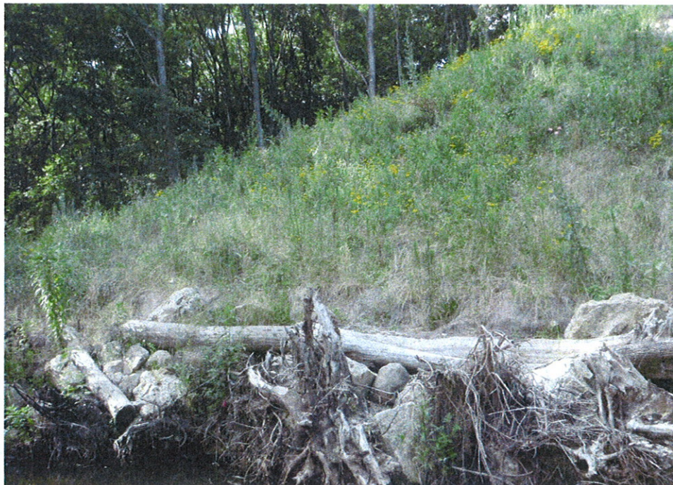
Image 20 – Rootwad composite installed by JFNew on Pheasant Branch Creek in the City of Middleton - 2008
