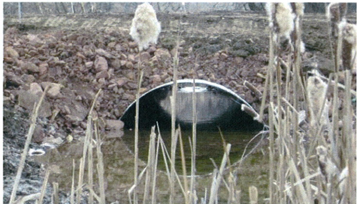
Image 17 – Example of a squash pipe in channel
