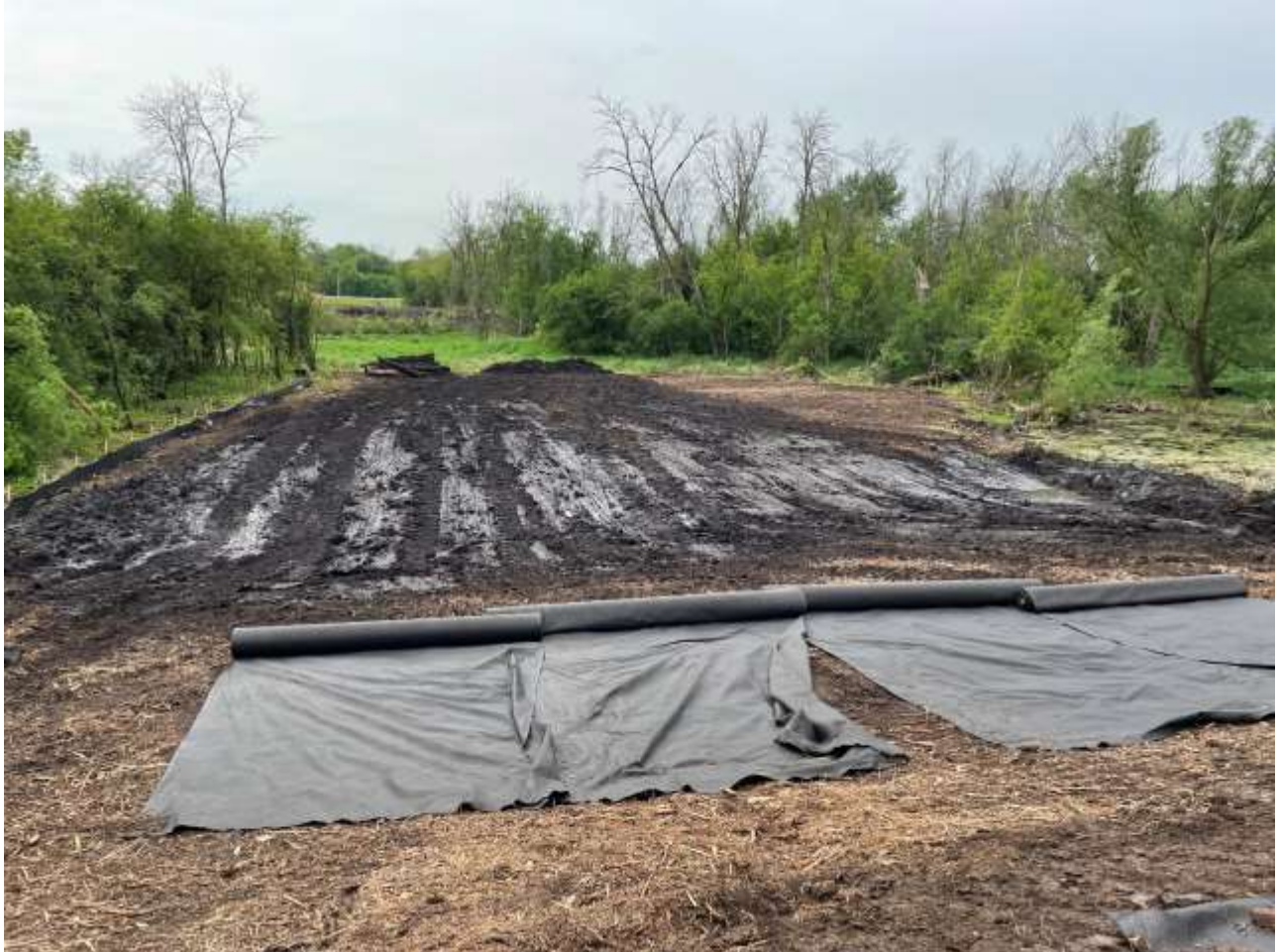
Northern portion of the project site (south of Chapel Hill Drive), cleared of vegetation, geotextile fabric laid out
