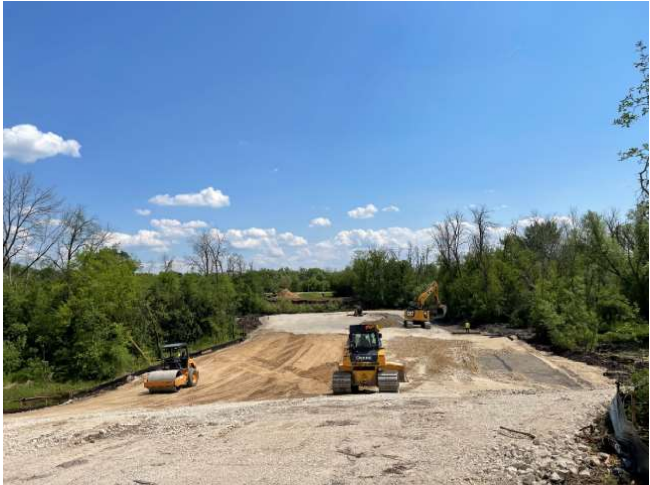
Northern portion of project site, installing the last layer of geogrid and select crushed material.
