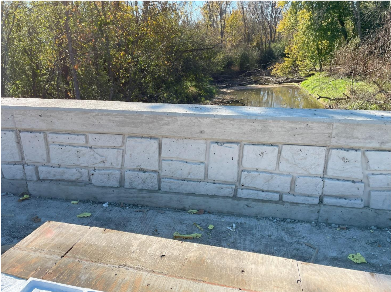
Parapet rock wall before sanding and grinding (touch up work and staining to occur in the spring).
