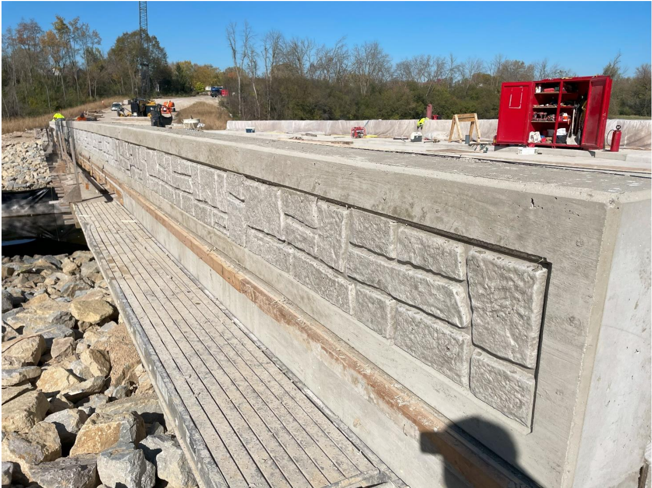
Parapet rock wall after sanding and grinding (touch up work and staining to occur in the spring).
