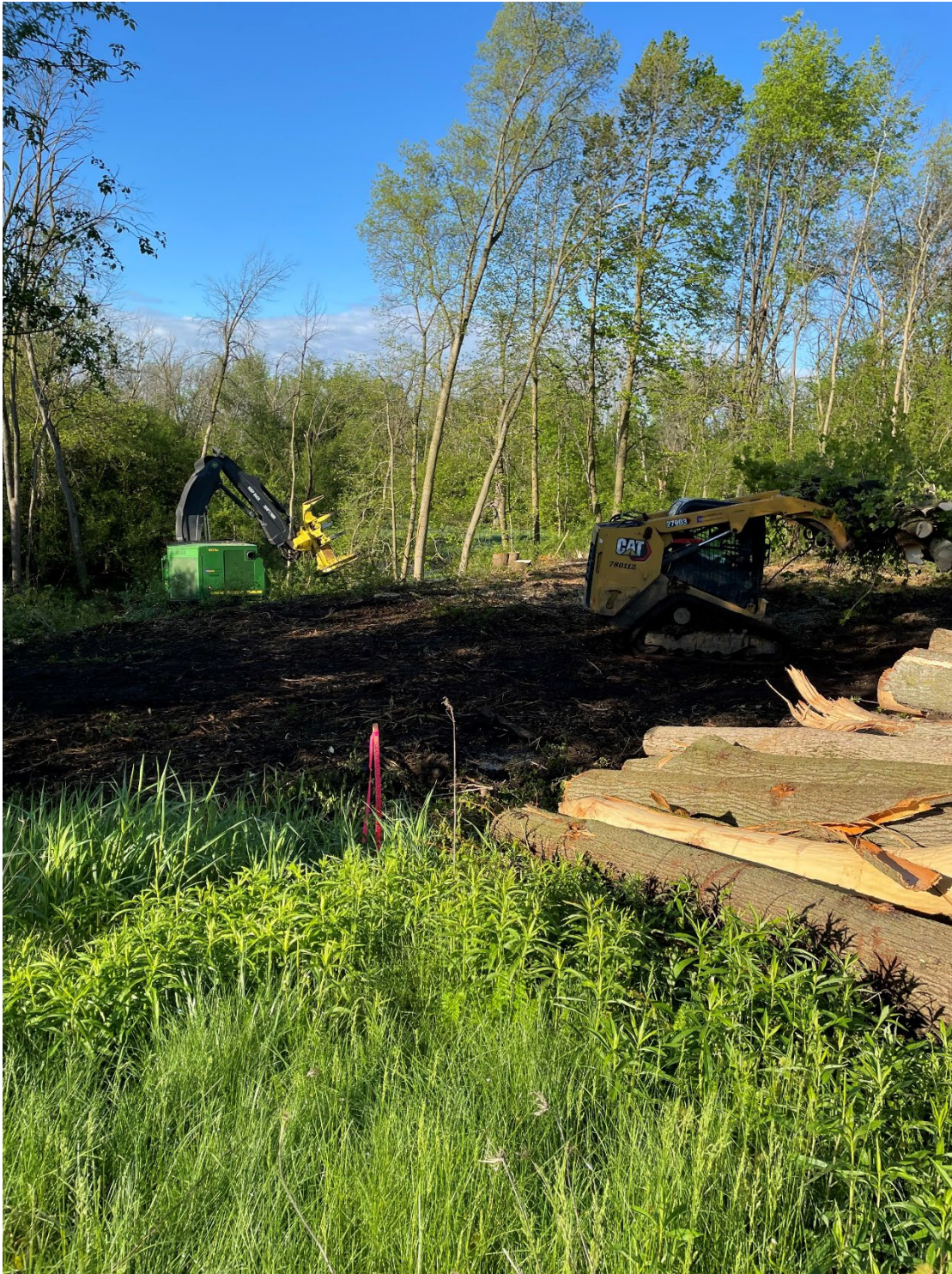
R.G. Huston clearing trees and vegetation in preparation for earthwork on the north portion of the project (south of Chapel Hill Drive).
